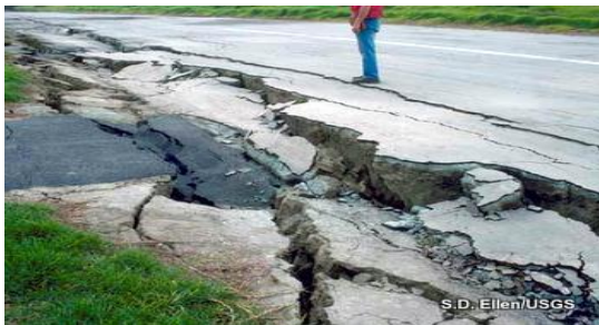
Fig-8- Effect of an Earthquake
